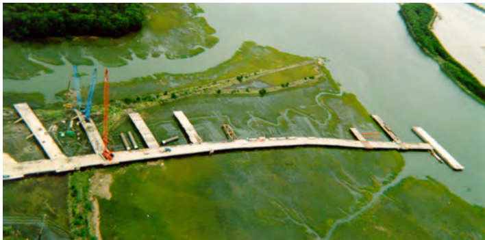
Figure 3.4-4. Award-winning effort to minimize wetland impacts on the Cooper River Bridge Project.
