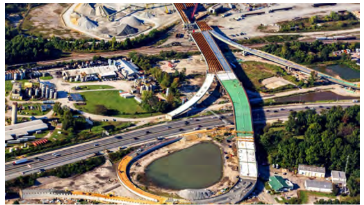
Figure 3.4-1. The ERT project has provided regional knowledge and working relationships to benefit the Team's quick start on I64HRB.
